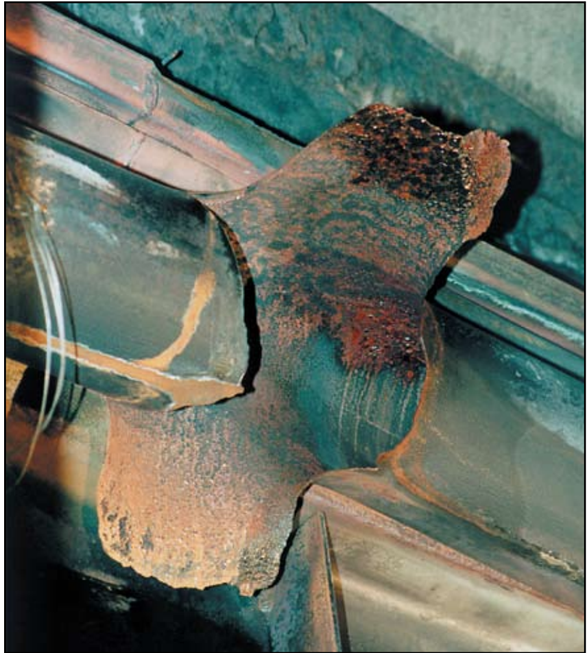
Figure 1: Rupture of a six-inch (152.4 mm) feedwater pipe in an area thinned by internal corrosion.
