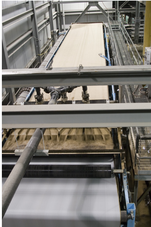
Figure 10 –Vacuum belt filter
